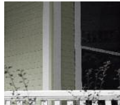
Trimworks beaded corner post.
